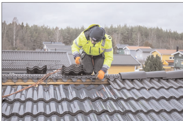
First installation of Bender SunWave roof tiles, incorporating Midsummer’s solar panel technology, on a townhouse outside Stockholm, Sweden.
