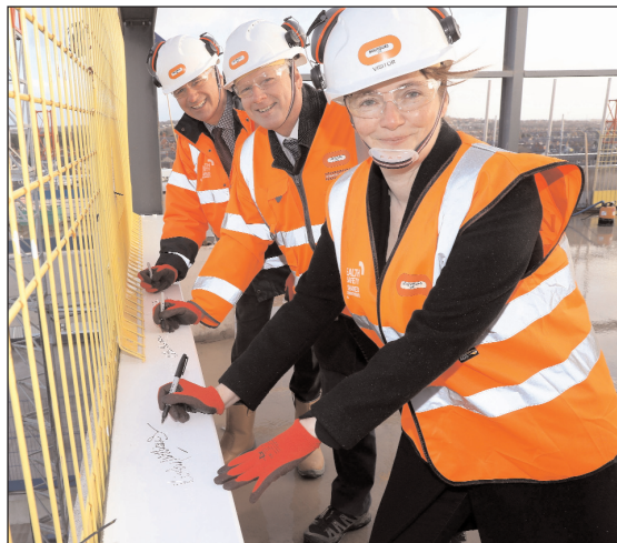
(r to l) Education Minister Kirsty Williams AM, Cardiff University president & vice-chancellor professor Colin Riordan and Bouygues UK's CEO Rob Bradley sign a beam to top out the Translational Research Facility.
